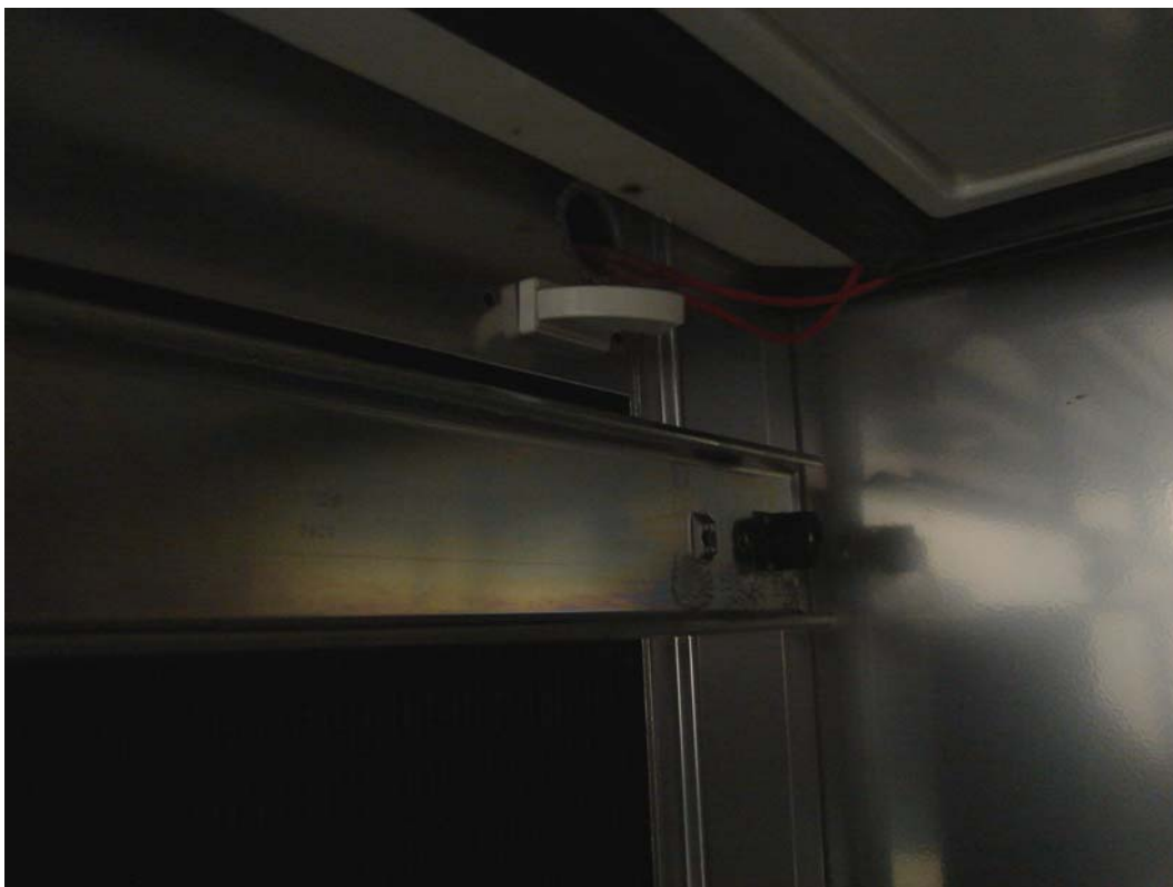
Figure 20: Heated seal wires and Inner wall penetration
